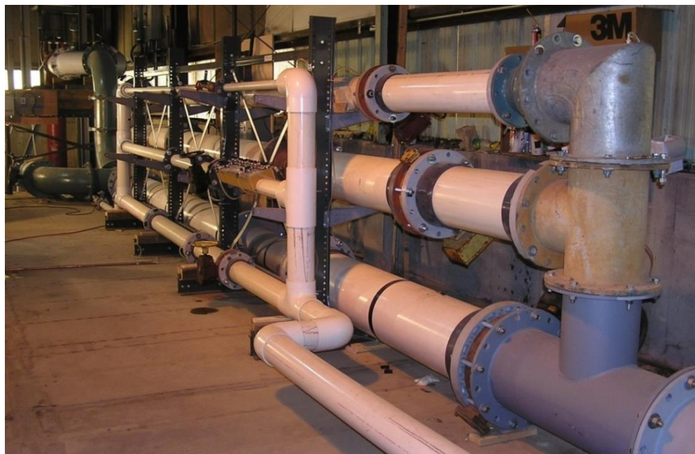
Figure 6: Photograph Showing Laboratory Flow Meters
