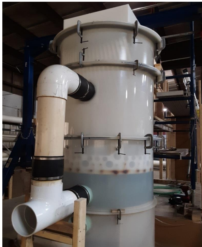
Figure 4: Outlet and Bypass Piping
