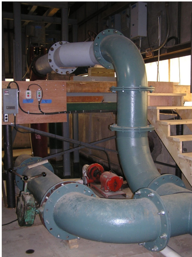
Figures 4 & 5: Test Loop Flow Meters and 50 HP Pumps
