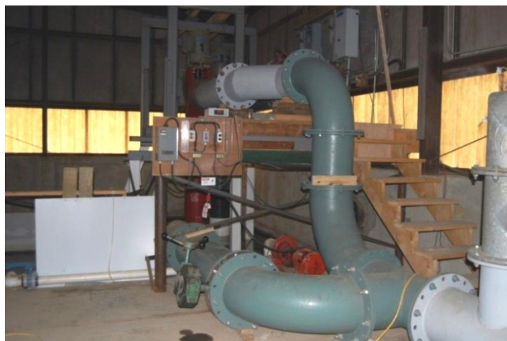
Figure 5: Photograph Showing Laboratory Pumps
